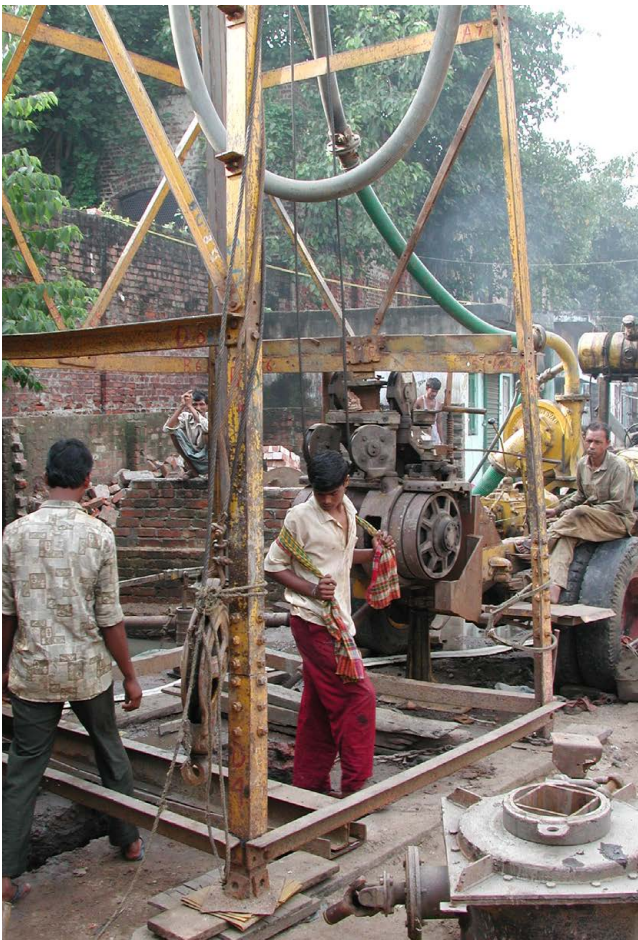
Water supply infrastructure, 2002
